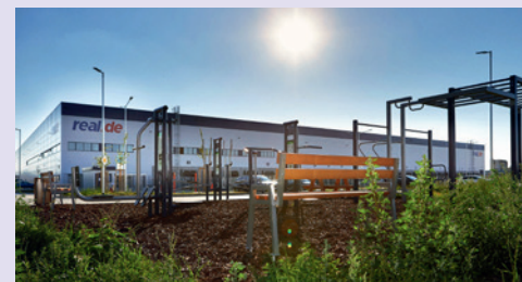
Construction also continues at Panattoni Park Cheb, where Panattoni is building a hall for fashion chain H&M – with 233,700 sqm, the largest logistics structure in CR
